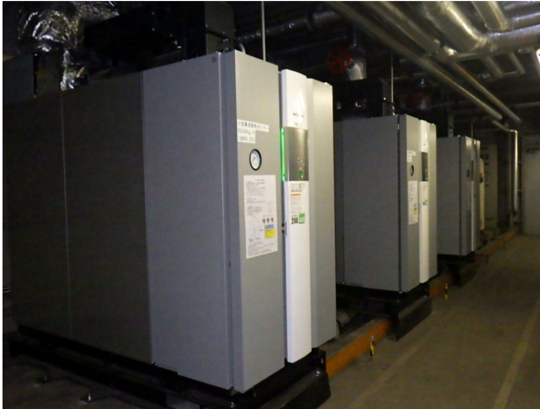
Boiler switched from kerosene to LNG fuel (Saijo Factory)
